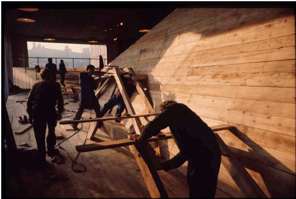
Figure 12. The practicable in Amiens under construction by a local company in collaboration with the cultural center's staff.
